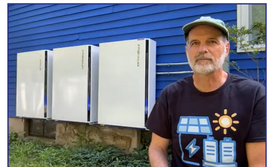
Andy is surrounded by solar panels on the roof of Brownstone Intermediate School and standing near the batteries at his home.
